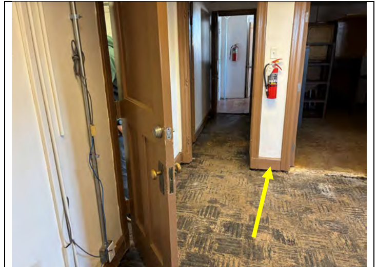
2. View of test #73 location (baseboard) with lead-based paint measured at 7.1 mg/cm 2 .
